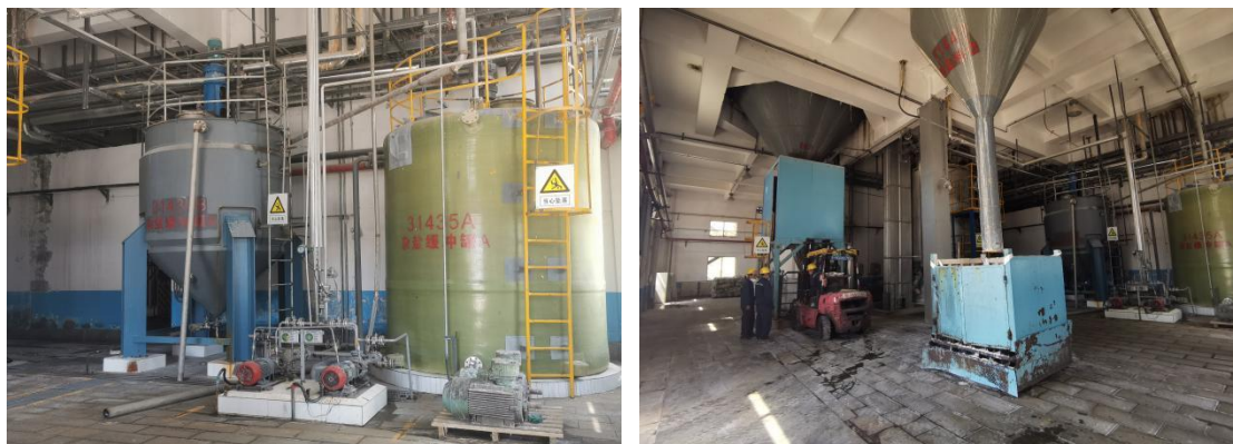
杂盐缓冲罐及杂盐料仓
